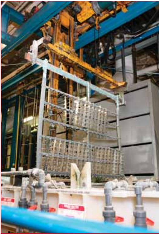
The plant boasts a world-class process that tin plates approximately 1 million pounds of aluminum and 2 million pounds of copper annually using environmentally friendly chemicals. Photo courtesy Schneider Electric/Square D
