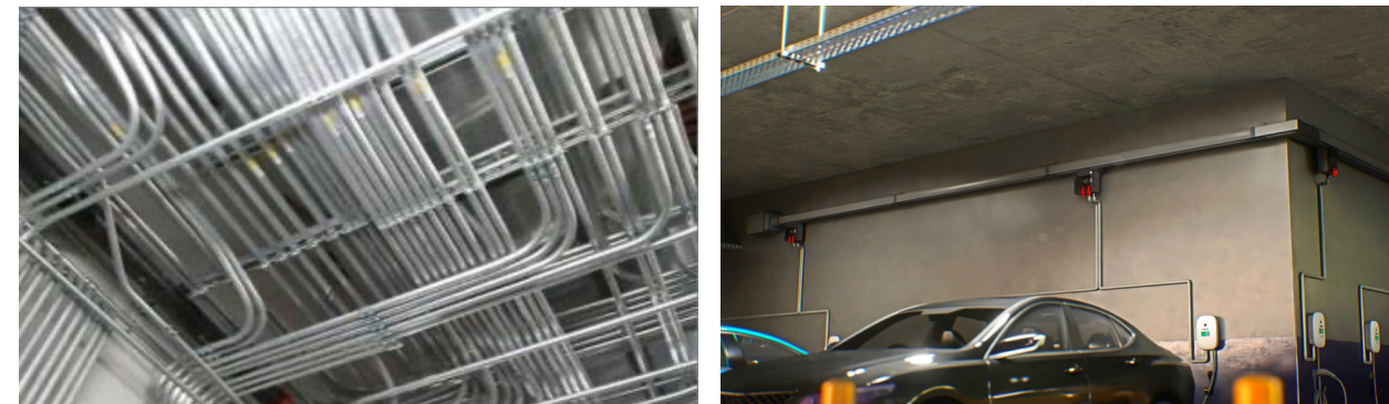
Figure 6. Conventional pipe & wire system (left) vs. track busway power distribution system (right)
